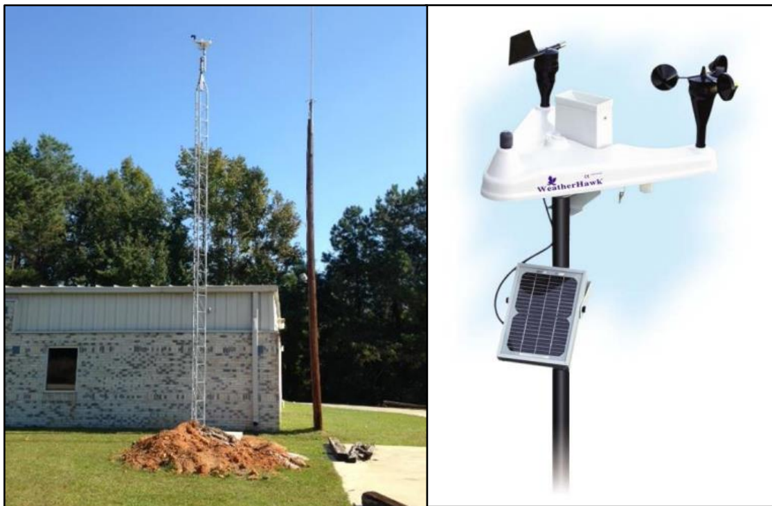
Figure 2.3 Typical RC Winds Station, Left- Example RC Winds Station, Right- WeatherHawk weather station, from K. Aucoin, and Campbell Scientific.
