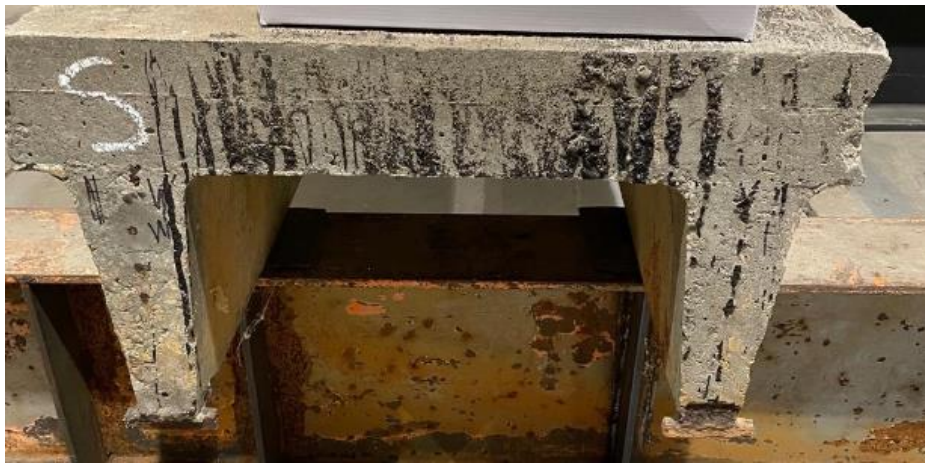
Figure A.7 C2 (NBI 9) end deterioration.
