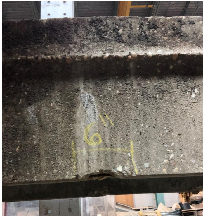
Figure A.38 C10 (NBI 2) small spall.
