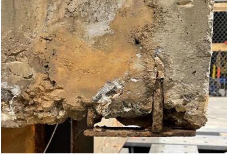
Figure A.12 C4 (NBI 4) moderate spall.
