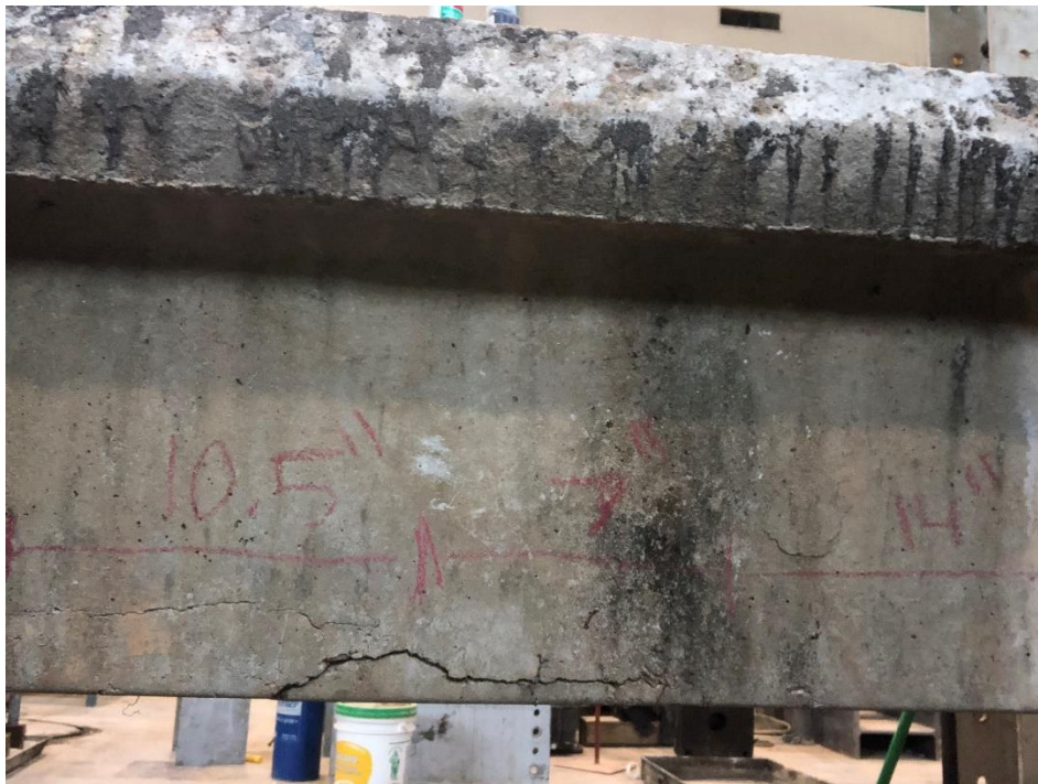
Figure A.49 C12 (NBI 4) wide crack near midspan.
