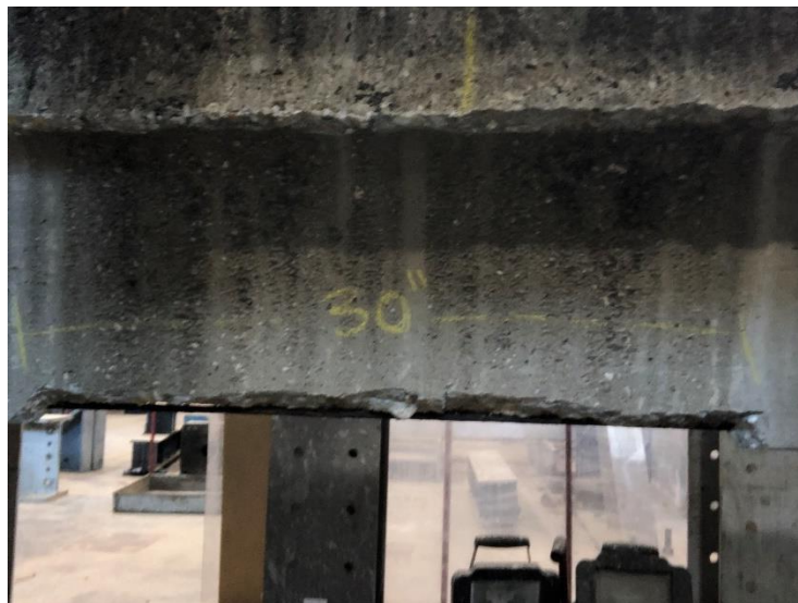
Figure A.31 C9 (NBI 3) major defect at midspan.
