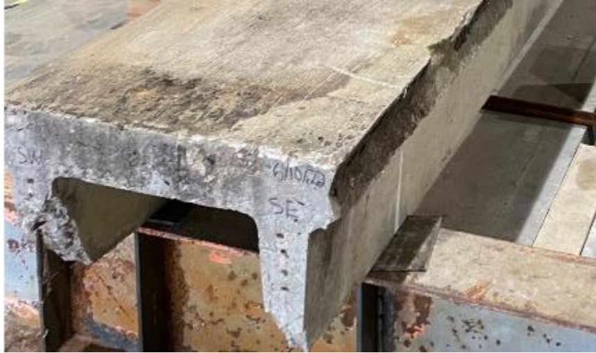
Figure A.4 C1 (NBI 7) end spalling, minor defect.
