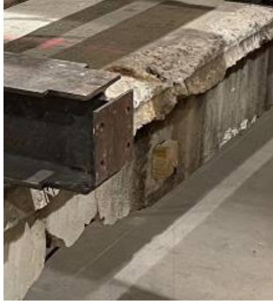
Figure A.19 C6 (NBI 1) severe deterioration.
