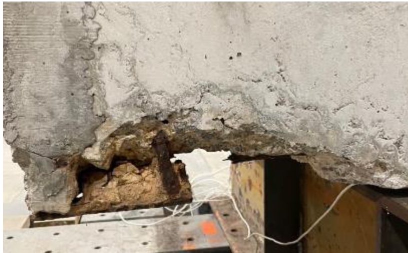
Figure A.13 C4 (NBI 4) moderate spall and corrosion.
