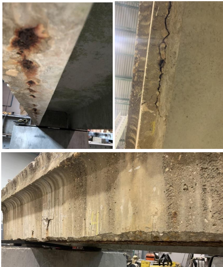
Figure 4.2 Examples of channel deterioration.
