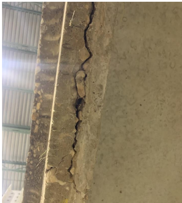
Figure A.25 C8 (NBI 3) wide crack.
