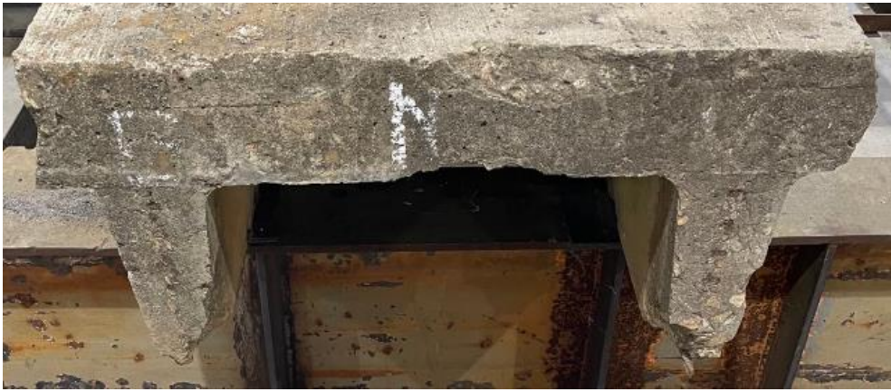
Figure A.10 C3 (NBI 7) end spalling.
