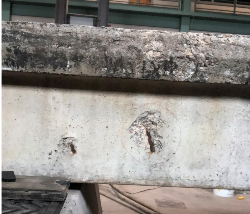
Figure A.42 C11 (NBI 6) small spalling.
