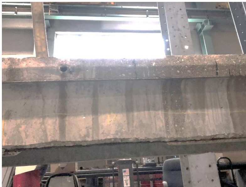
Figure A.39 C10 (NBI 2) major defect, severely compromised.
