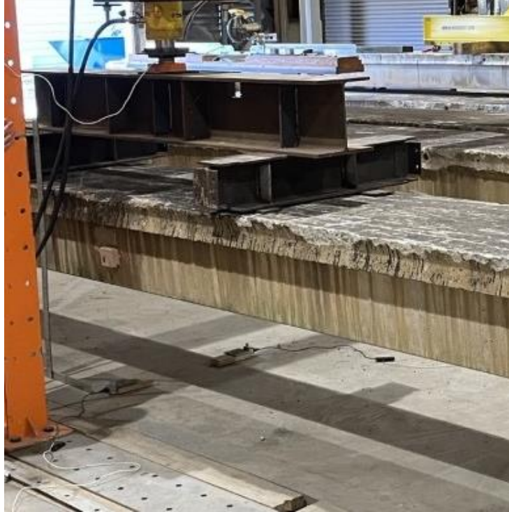
Figure A.21 C7 (NBI 6) flange spalling.
