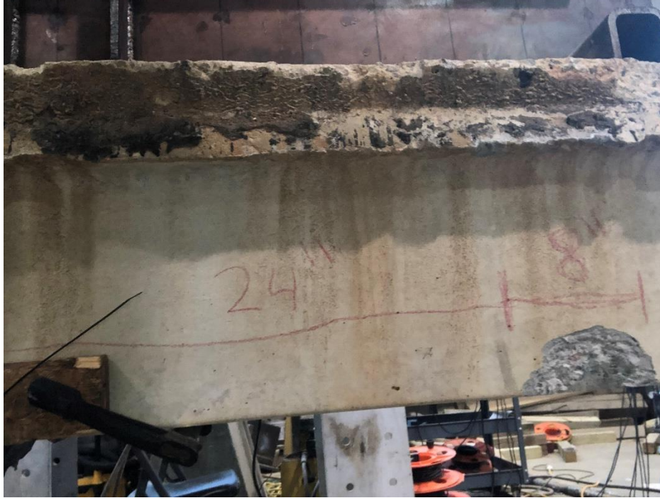
Figure A.46 C11 (NBI 6) large spall near midspan.
