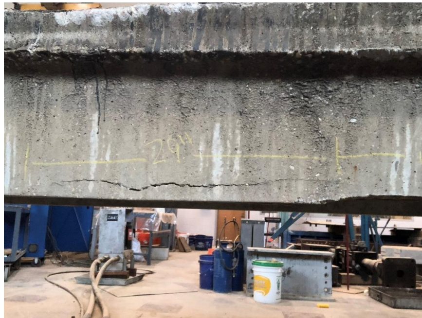
Figure A.29 C9 (NBI 3) moderate defect near quarter span.
