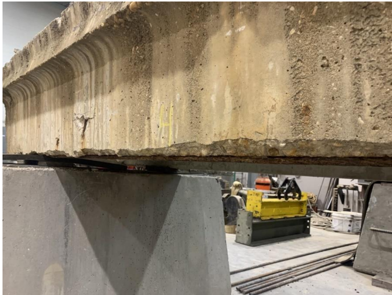
Figure A.22 C8 (NBI 3) major defect.
