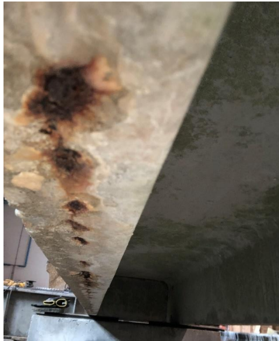
Figure A.41 C10 (NBI 2) rust staining, moderate defect.
