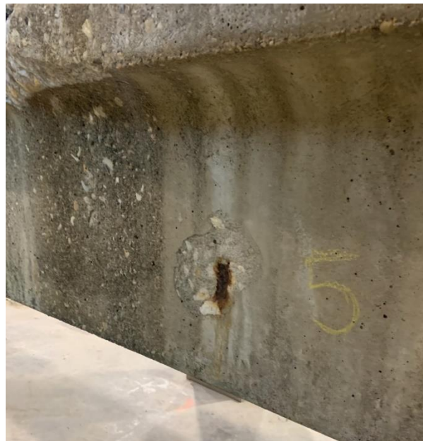
Figure A.27 C8 (NBI 3) minor defect.
