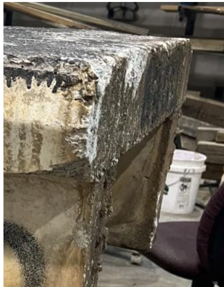
Figure A.53 C13 (NBI 7) flange spalling.
