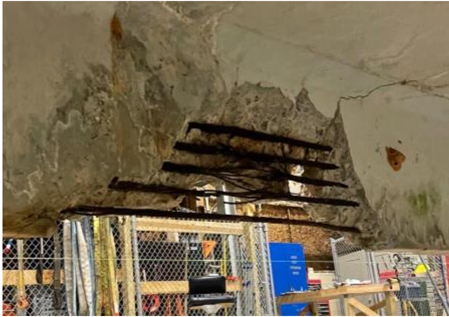
Figure A.18 C6 (NBI 1) imminent failure at midspan.
