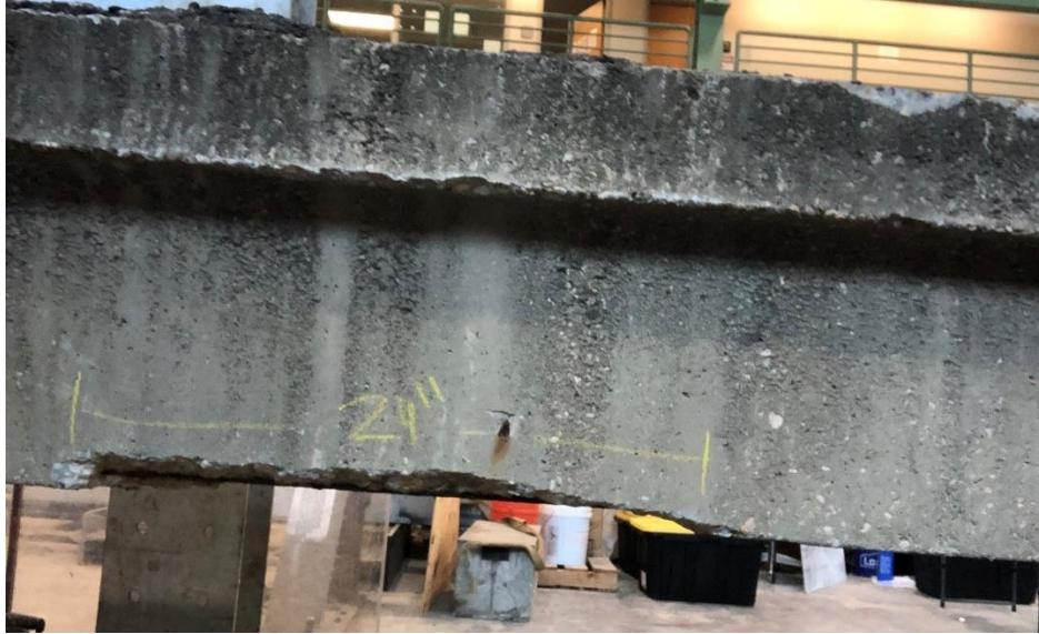
Figure A.32 C9 (NBI 3) major defect near midspan.
