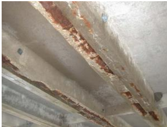
Figure 2.1 Typical PCB deterioration (Klaiber et al. 2003).
