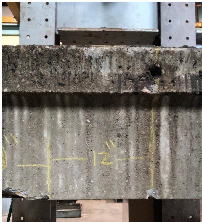
Figure A.37 C10 (NBI 2) small spall.
