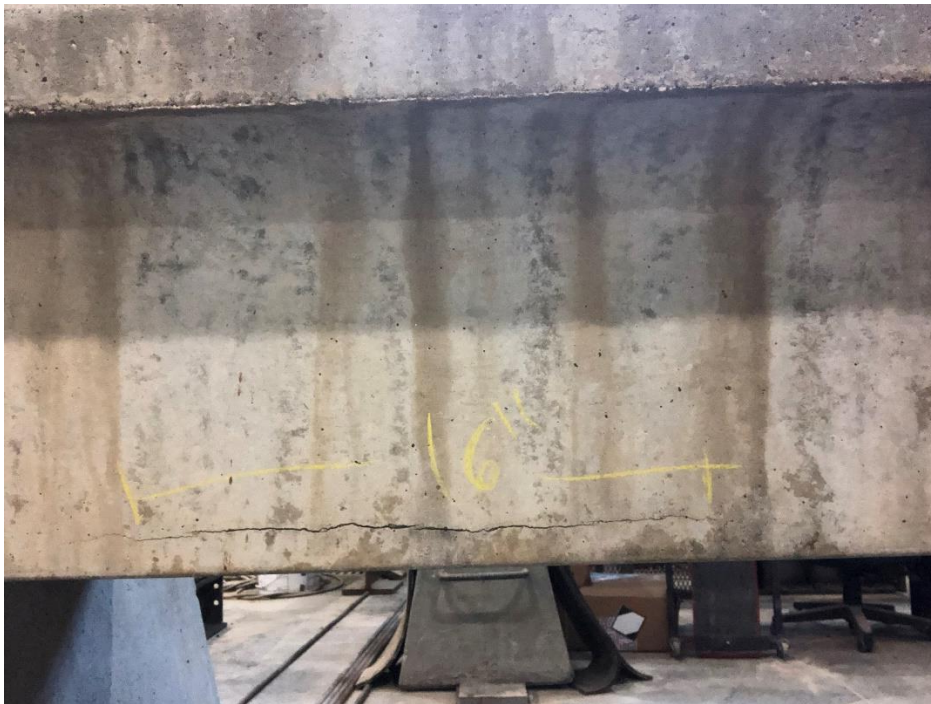
Figure A.35 C10 (NBI 2) medium crack.
