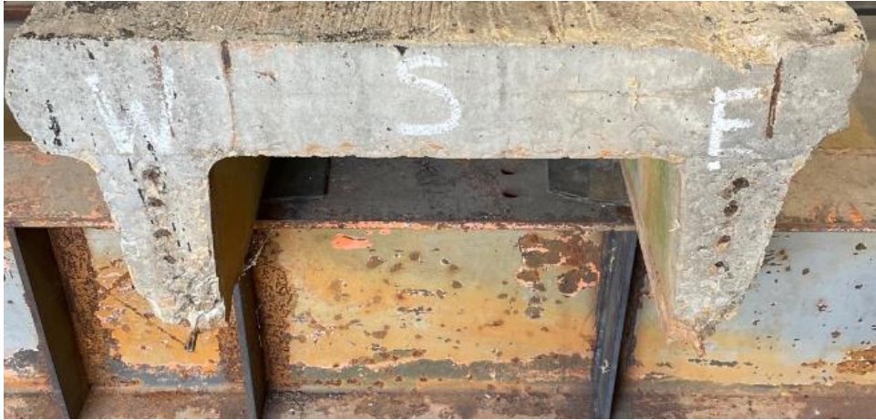
Figure A.11 C3 (NBI 7) exposed strands.
