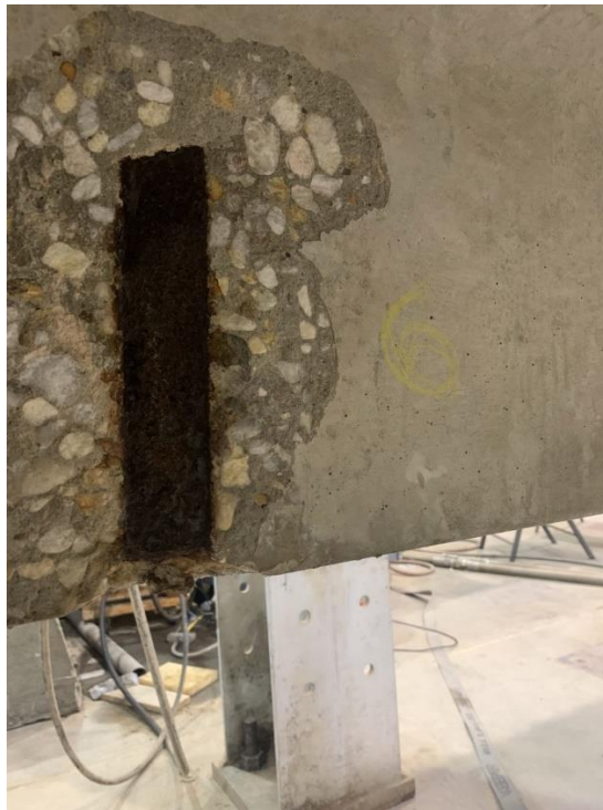
Figure A.23 C8 (NBI 3) moderate spall.
