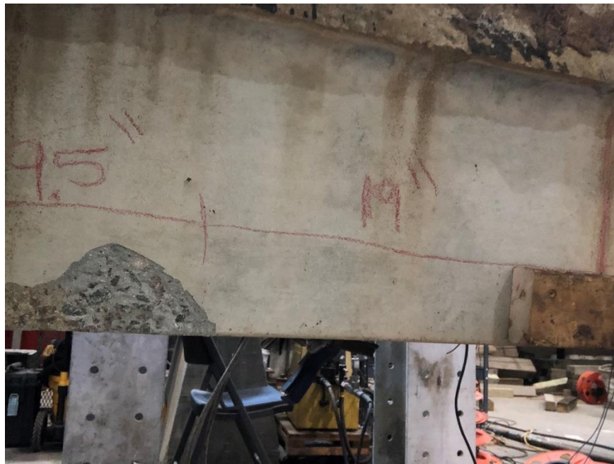
Figure A.47 C11 (NBI 6) large spall near midspan.
