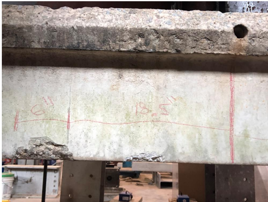
Figure A.43 C11 (NBI 6) small spalling near midspan.
