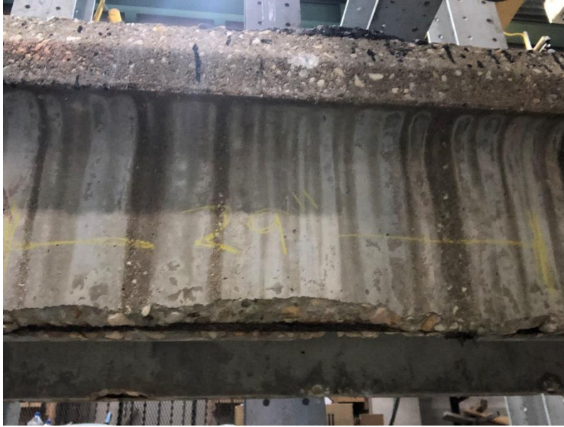
Figure A.40 C10 (NBI 2) major defect.
