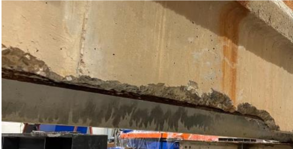
Figure A.16 C5 (NBI 3) major defect near load point.
