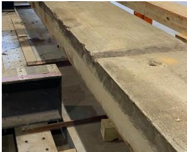
Figure A.9 C3 (NBI 7) flange spalling.
