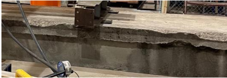
Figure A.6 C1(NBI 7) flange spalling, minor defect.
