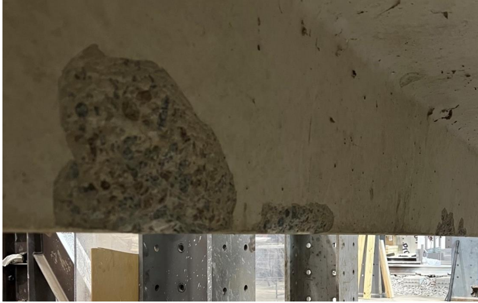
Figure A.50 C12 (NBI 4) large and small spalling.
