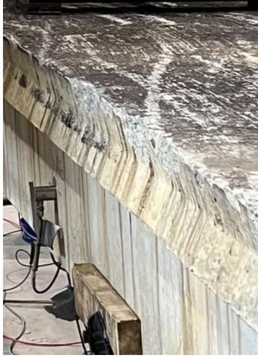
Figure A.52 C13 (NBI 7) flange spalling.
