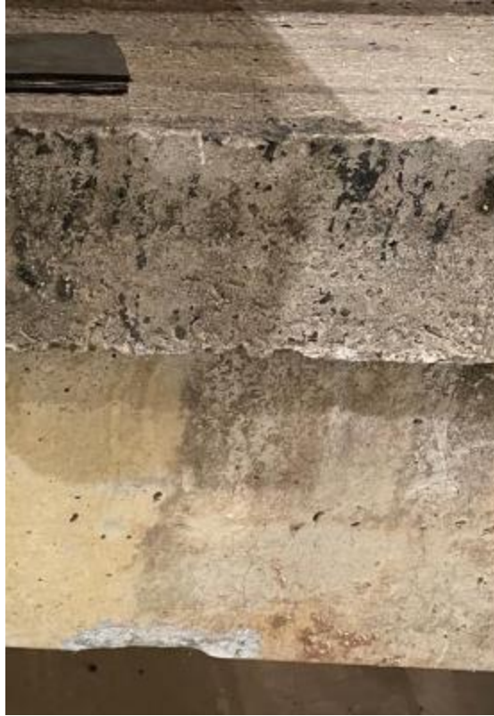
Figure Error! Use the Home tab to apply 0 to the text that you want to appear here. A.8 C2 (NBI 9) inherent defect.
