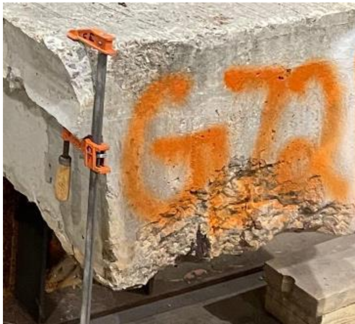
Figure A.15 C5 (NBI 3) large spalling, moderate defect.
