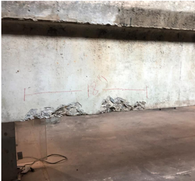
Figure A.44 C11 (NBI 6) small spalling.
