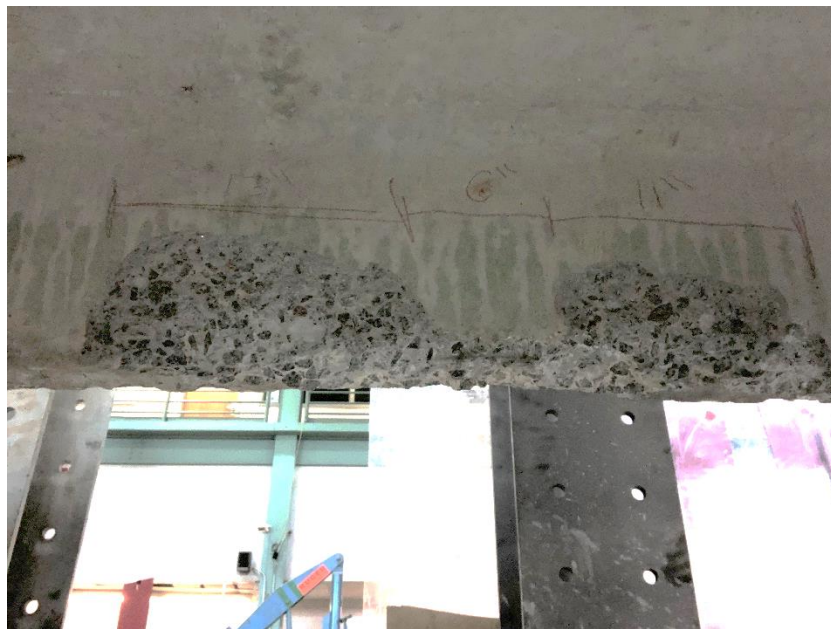
Figure A.45 C11 (NBI 6) large spalling.
