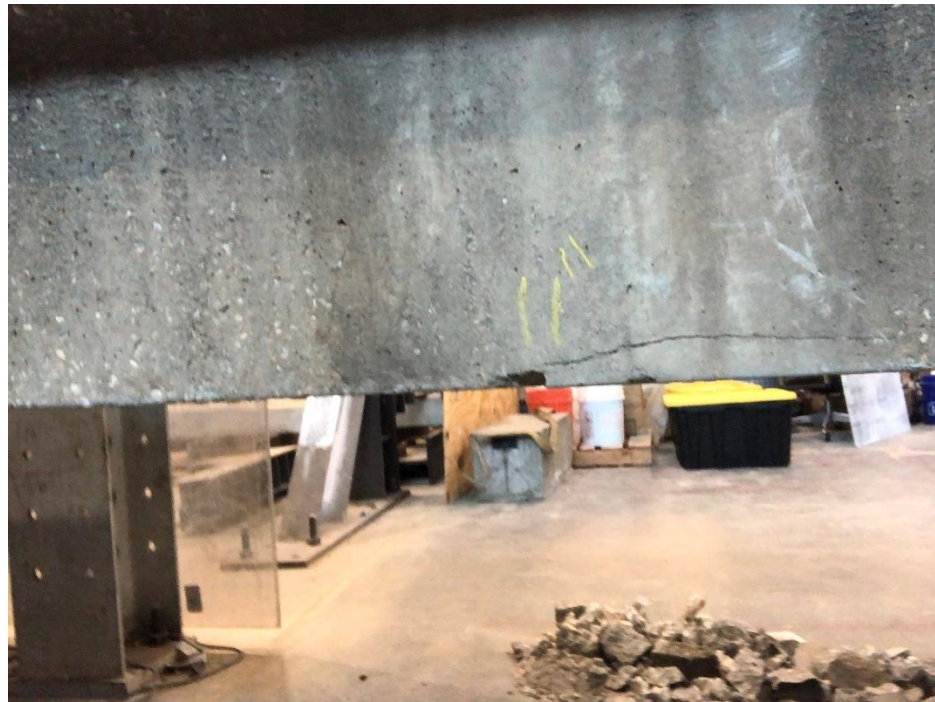
Figure A.33 C9 (NBI 3) medium crack, minor defect.
