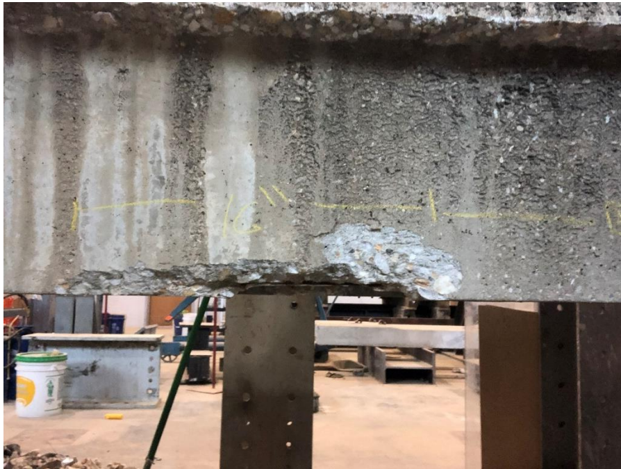
Figure A.30 C9 (NBI 3) moderate defect near midspan.
