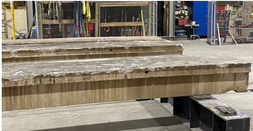
Figure A.20 C7 (NBI 6) widespread minor defects.
