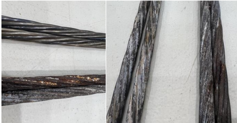
Figure 4.1 Various levels of strand corrosion.
