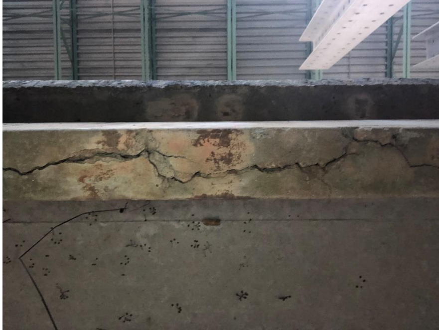
Figure A.48 C12 (NBI 4) wide crack, moderate defect.
