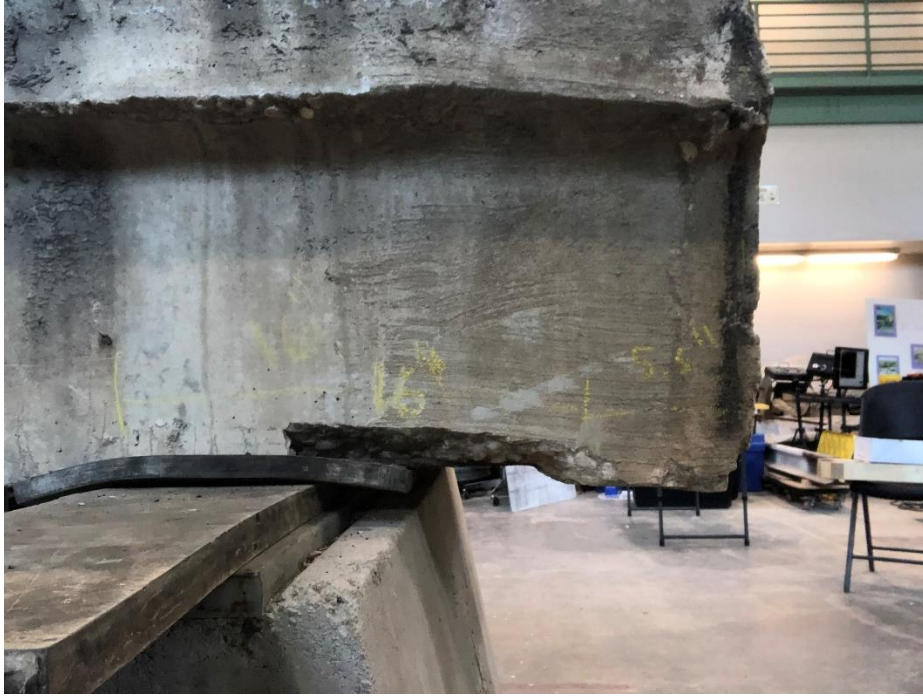
Figure A.34 C9 (NBI 3) large spall.
