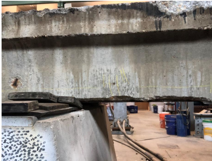
Figure A.28 C9 (NBI 3) major defect.
