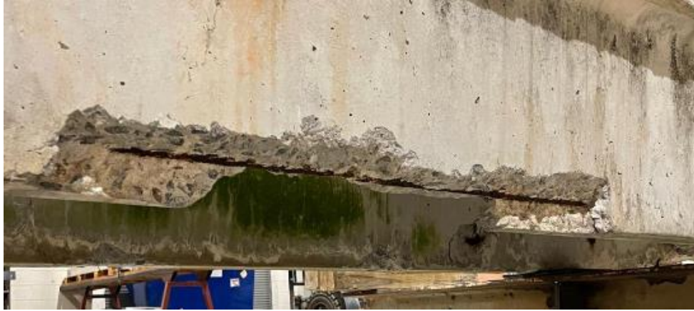
Figure Error! Use the Home tab to apply 0 to the text that you want to appear here.A.14 C4 (NBI 4) major defect near quarter span.
