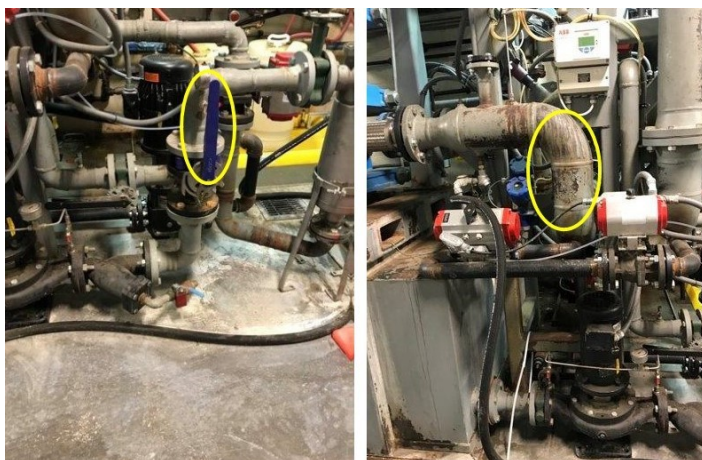
Figure 2. Potential sites for valves: tower water side (left) and antifreeze side (right).
