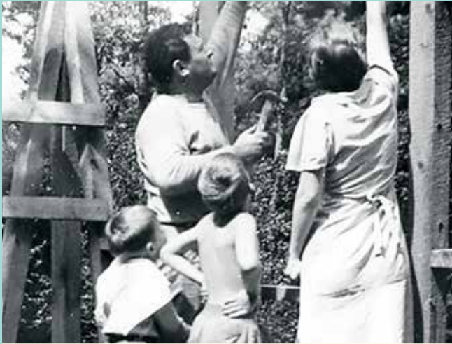
Robert and Virginia Bass work on a building project at the Saluda house, supervised by their sons George (left) and Robert (Bobby).
