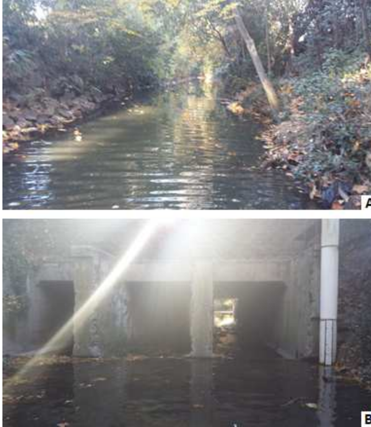
Figure A.13. At-Pickens Gage Site Cross Section. (A) View upstream from Pickens Street Bridge. (B) View downstream towards bridge box culverts with stilling well of gage on the right bank
