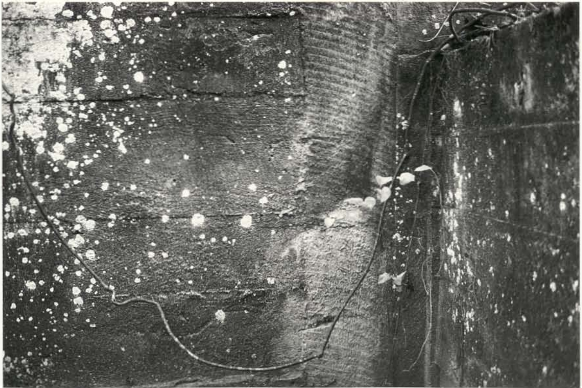
FIGURE 3. Impressions of Lumber Forms on Concrete at 38CL28.
