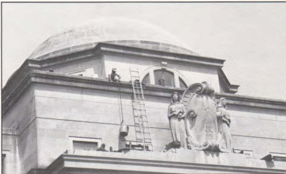
Workers race the clock to beat the summer heat in finishing repairs to McKissick's roof.
