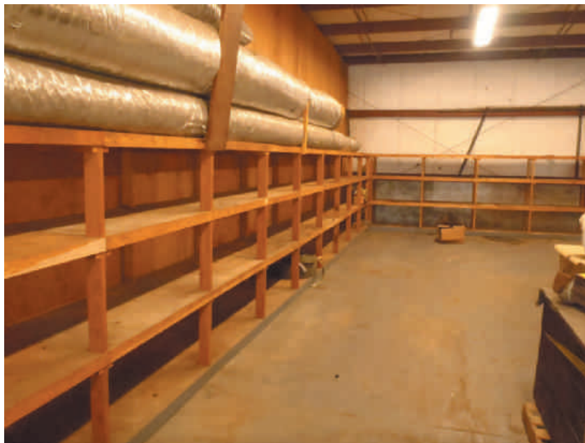
Another view of new curation facility space prior to renovation. (SCIAA photo)
